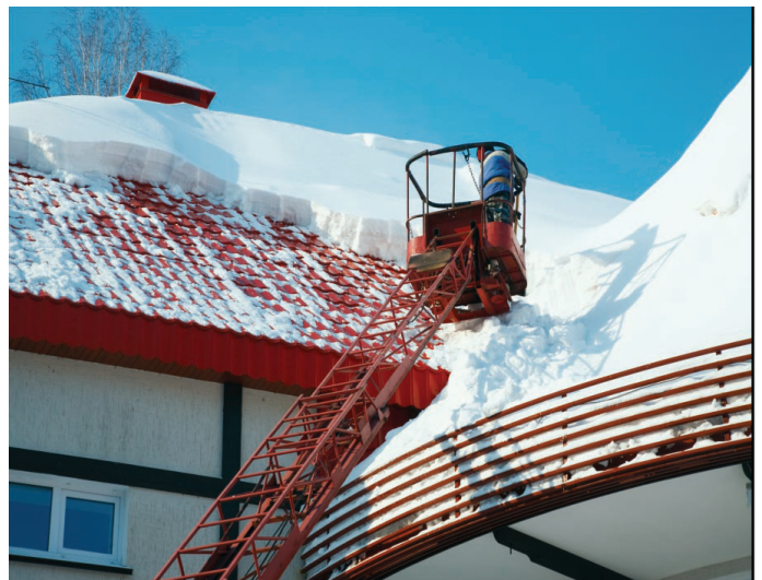
An aerial lift is being used in a snow removal operation. The worker is using a restraining belt and lanyard for protection.
